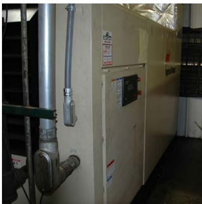
Air Compressor Control
