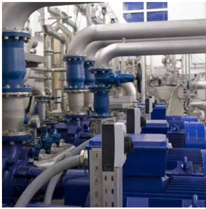
Industrial Pump Control
