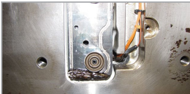
Actual Leak Detected with Alarm
